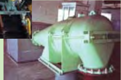
Heavy media cyclone
